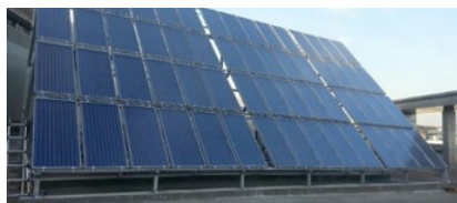
(Suwon DC) Solar Water Heating System
