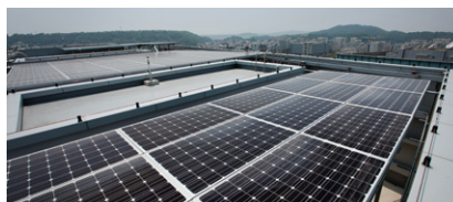
(Sangam DC) Photovoltaic Power Generation
