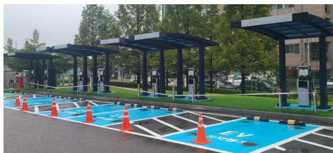
Suwon DC EV Charging Stations
