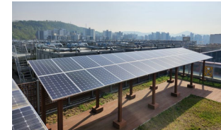
Sangam Data Center Solar Power Generation Facility
