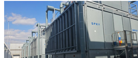
Suwon DC Cooling Tower (open-type)
