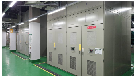
Suwon DC Transformer
