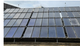
Suwon Data Center Solar Water Heating System
