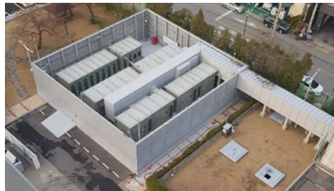
Existing outdoor power distribution room
