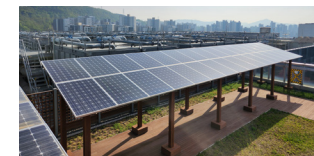
Sangam DC Photovoltaic Power Generation
