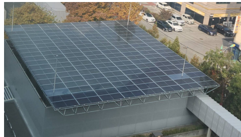
Outdoor power distribution room after installing solar power generation facilities
