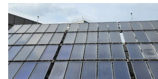
Suwon DC Solar Water Heating System
