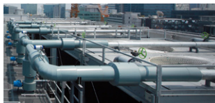
Sangam DC Cooling Tower
