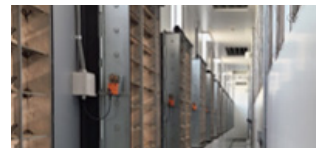
Outdoor Air Damper
