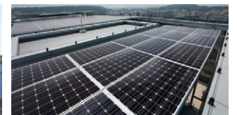
Sangam DC Photovoltaic Power Generation
