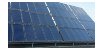
Suwon DC Solar Water Heating System
